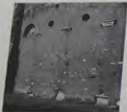
Fig. 177. S. Stepha. Rotunda. Southwest sector, section showing lower and upper tubular masonry wall (upper formed with tubular masonry).
